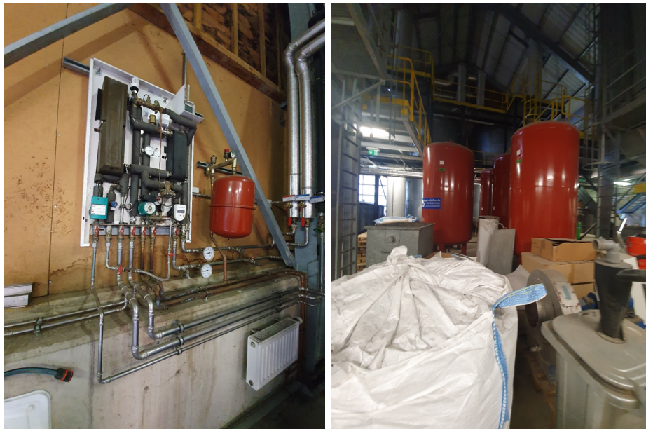
Figure 3 – Different pictures of the Biomethanisation and the Wood chip heating plant of the district heating network.
